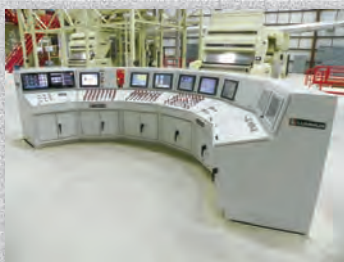
Controls and Control Systems
